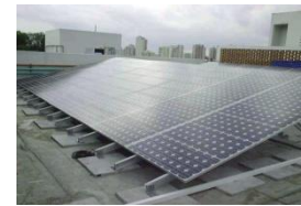
SP PV system
