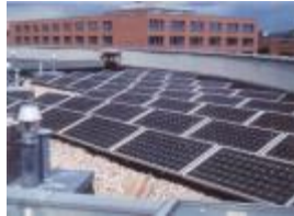
PUB PV system
