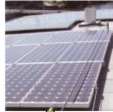
HDB PV system
