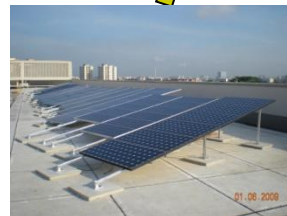
SP PV system
