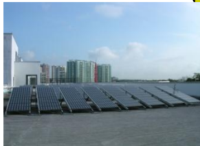
SP PV system
