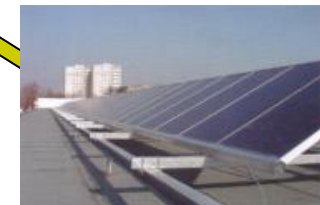
Other PV system
