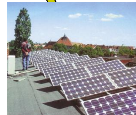
Other PV system
